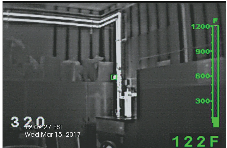
2. Distinction of hot water pipes in a boiler room.
